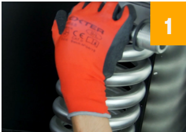
CLEANING THE COIL.
